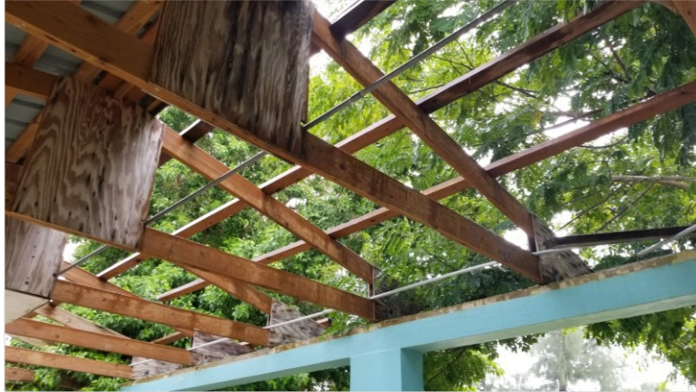
Figure 9: Roof panel blew off purlin nailers.
