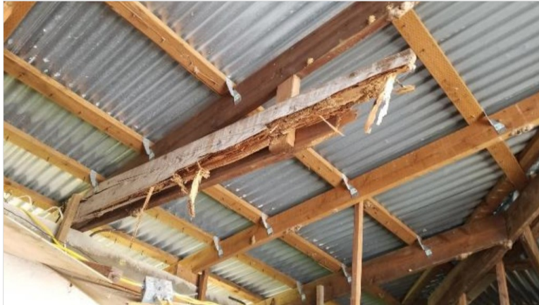
Figure 7: Roof framing showing lack of structural roof deck under corrugated metal roof, rafters spaced too far apart, informal connectors from rafters to walls, and extensive termite damage to most roof structural members.
