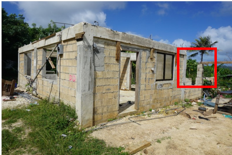
Figure 4: Home with concrete frame with CMU in-fill wall construction. The CMUs have variable joint spacing down to no joint spacing. Rafter connectors are informal and spaced far apart. The back-right wall of the house (in red box) has been blown off with the roof and is separated from the home.
