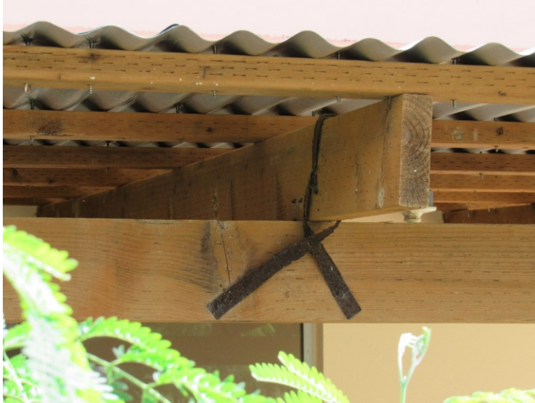
Figure 5: Wood-framed roof-to-beam construction. Connection is an informal method that is not an engineered solution.
