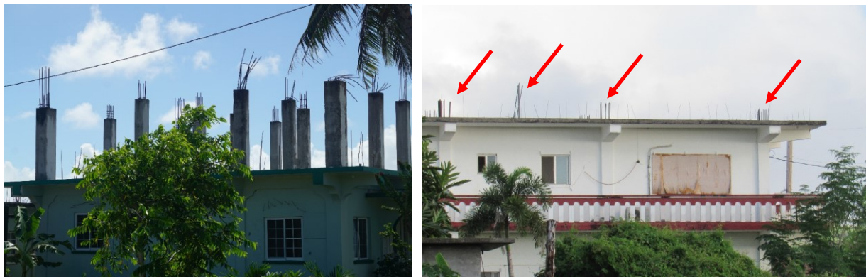
Figure 2: Red arrows indicate “Hope sticks” extending out from base home construction. These unprotected reinforcing bars will lead to damage of the base structure as they experience harmful corrosion.
