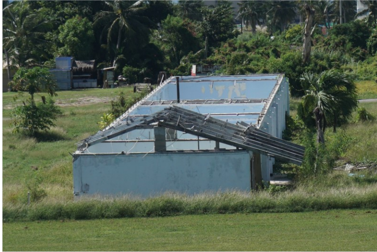
Figure 3: Building with entire roof blown off.
