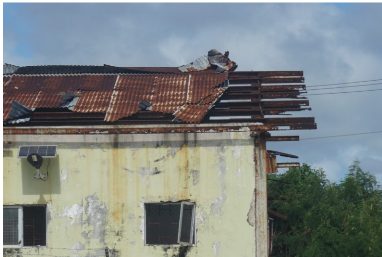
Figure 10: Corroded roof panel with zinc galvanizing consumed.
