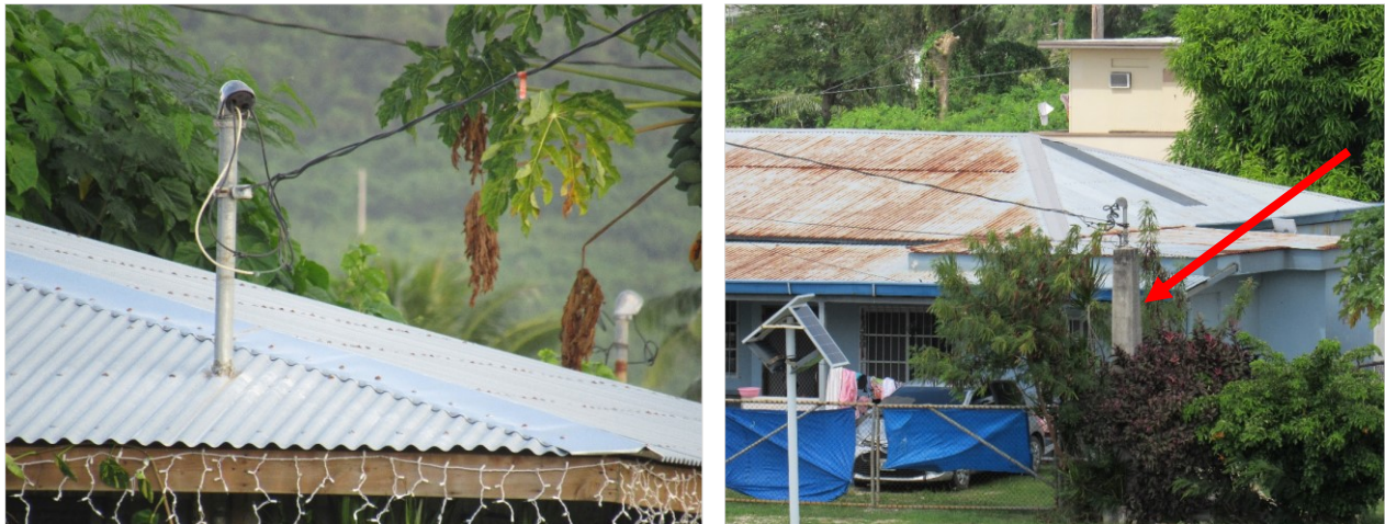
Figure 8: Left—Electric service mast going through roof; Right—Electric service on separate pedestal.
