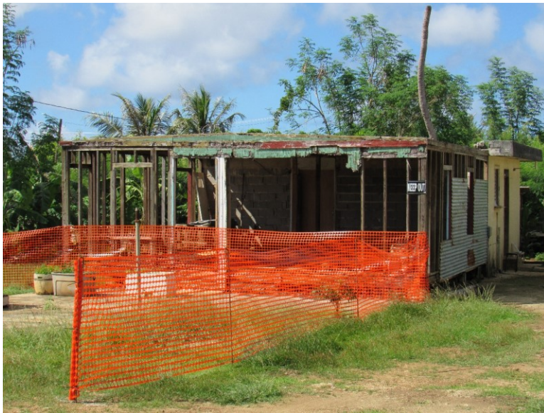
Figure 6: Wood-framed home that suffered near complete damage.
