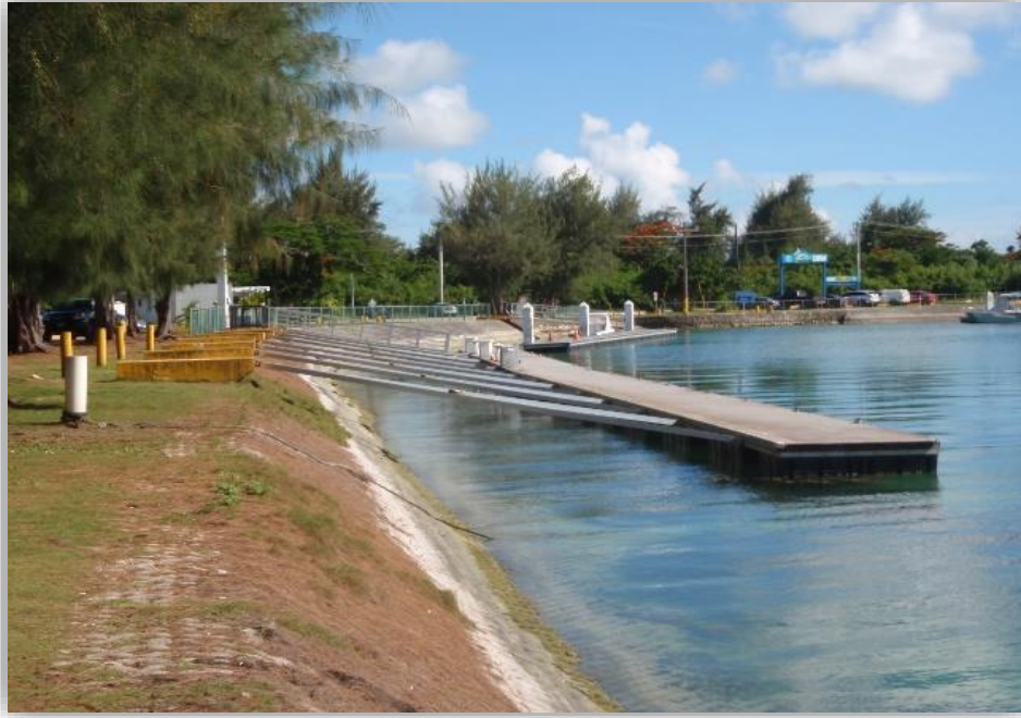
Figure 7.5 The resilient design at Smiling Cove Marina, Saipan helps dissipate wave energy to reduce shoreline erosion and promotes recreation in open space.
