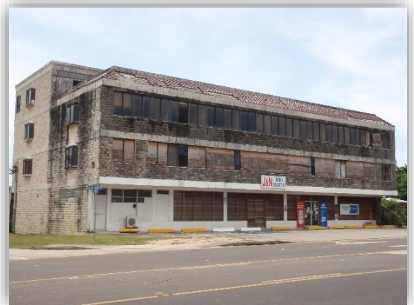
Figure 6.2 Abandoned since the 1990s, with progressive deterioration mainly from typhoons.
