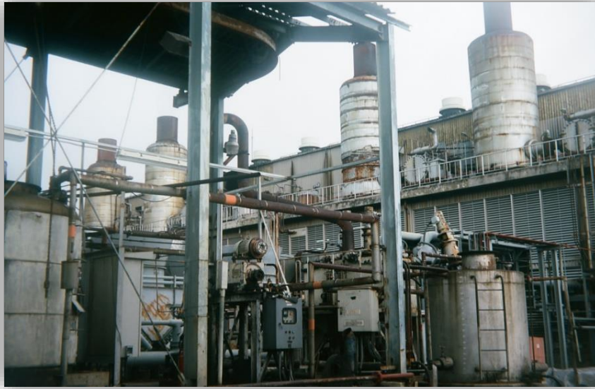
Figure 7.3 CUC Diesel Power Plant No. 1.
