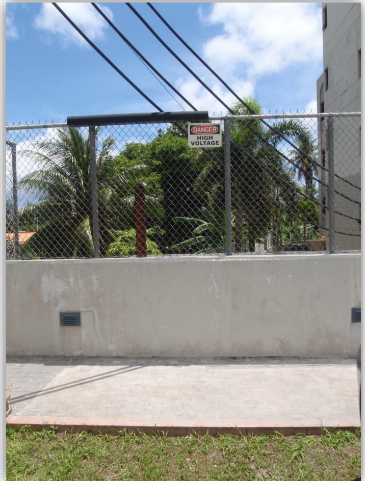
Figure 7.1 Insulator on steel fence at powerline contact. Not smart. Not safe.
