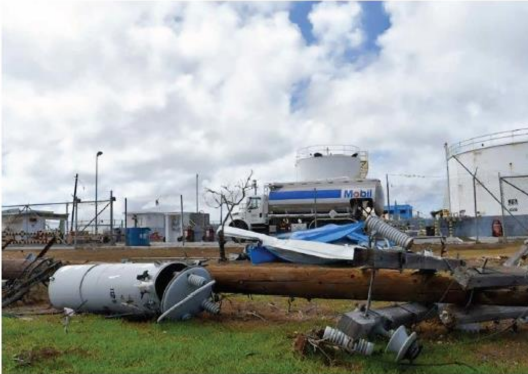
Electric and communications infrastructure downed and damaged by Typhoon Yutu. Photo by FEMA, 2018, courtesy of CNMI Office of Planning and Development.
