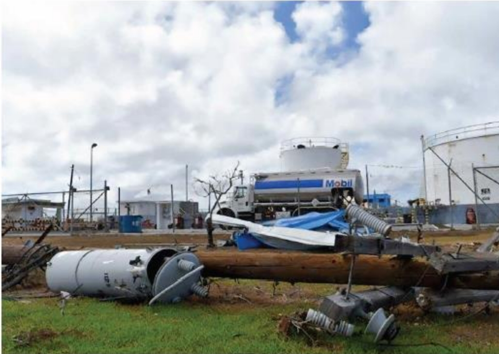
Electric and communications infrastructure downed and damaged by Typhoon Yutu. Photo by FEMA, 2018, courtesy of CNMI Office of Planning and Development.
