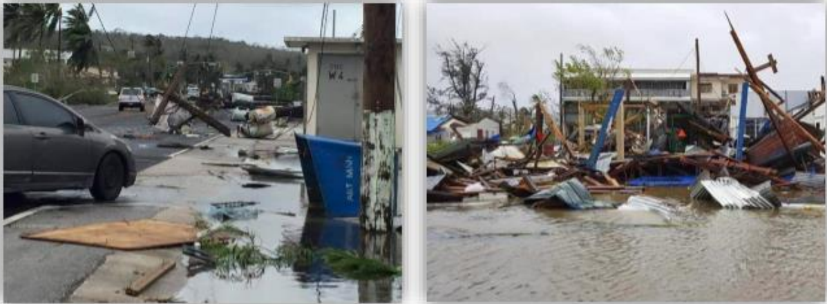
Figure 3.1 Storm-damage to the power distribution system from Super Typhoon Soudelor (left) and wreckage from Super Typhoon Yutu (right).
